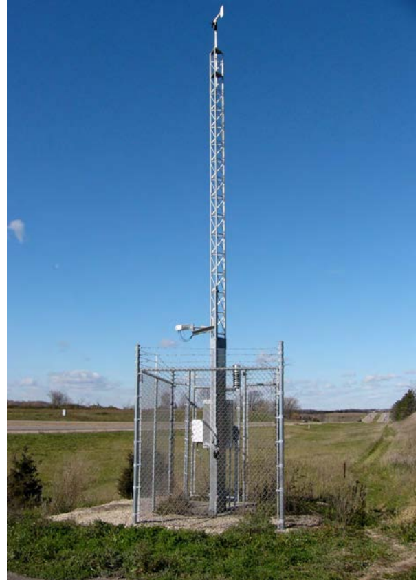
A roadside weather station.
