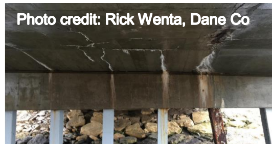
Rusting and concrete damage caused by corrosion from chlorides
